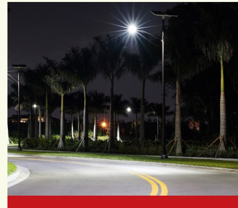
Solar Lights & Power Backup
